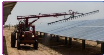
Innovation in Module Cleaning System (Semi - Automatic)
